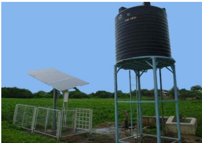
Well pumping with elevated storage tank
